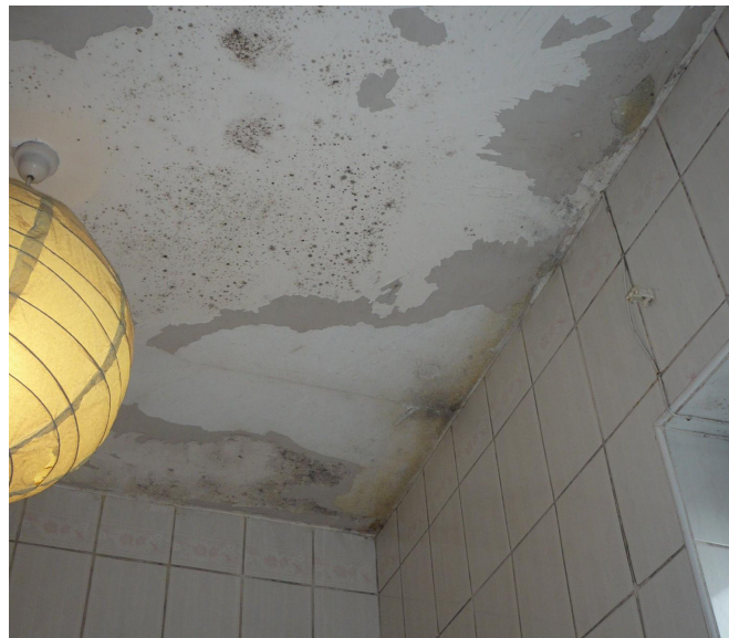
Figure 4: mould visible in the shower room where Figure 3 was measured
