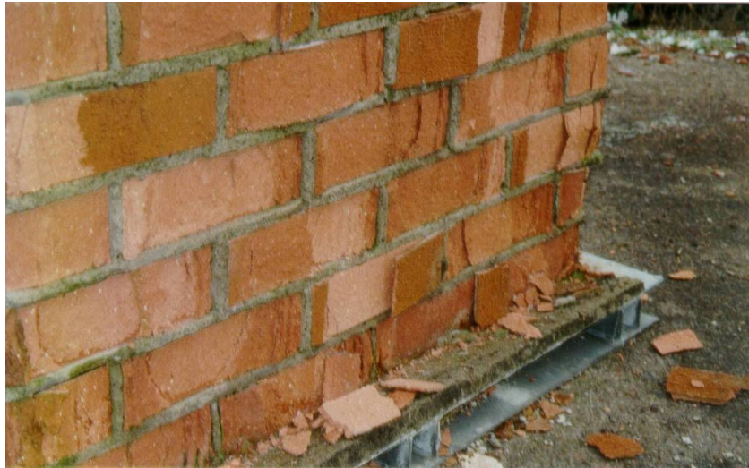
Figure 8: showing damage due to the freeze-thaw cycle can do to a solid brick wall Image courtesy of the Fraunhofer Institute, IBP Holzkirchen
